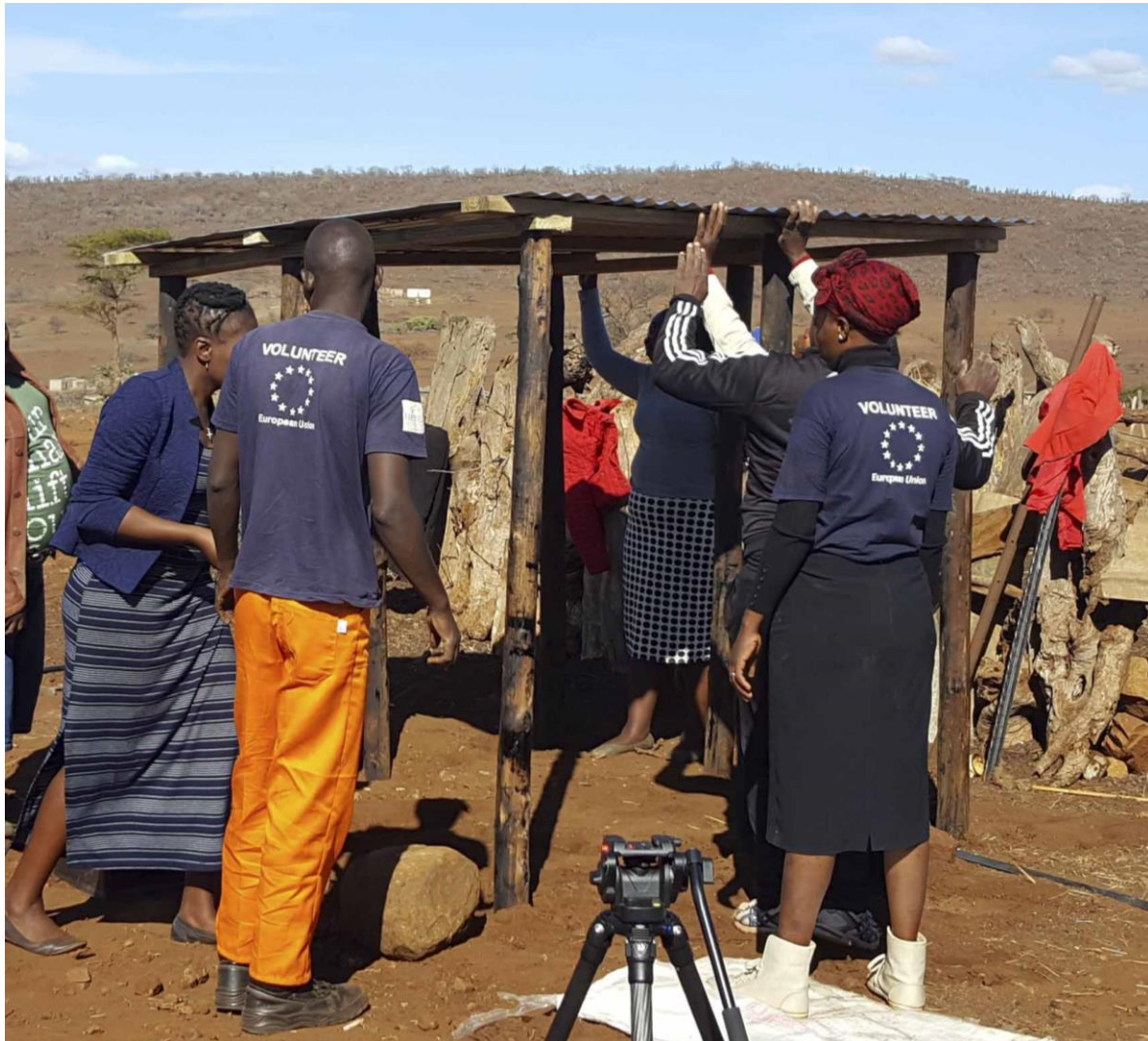
Community Animal Health Workers and staff in Jozini building an enclosure for goat kids' feeding
